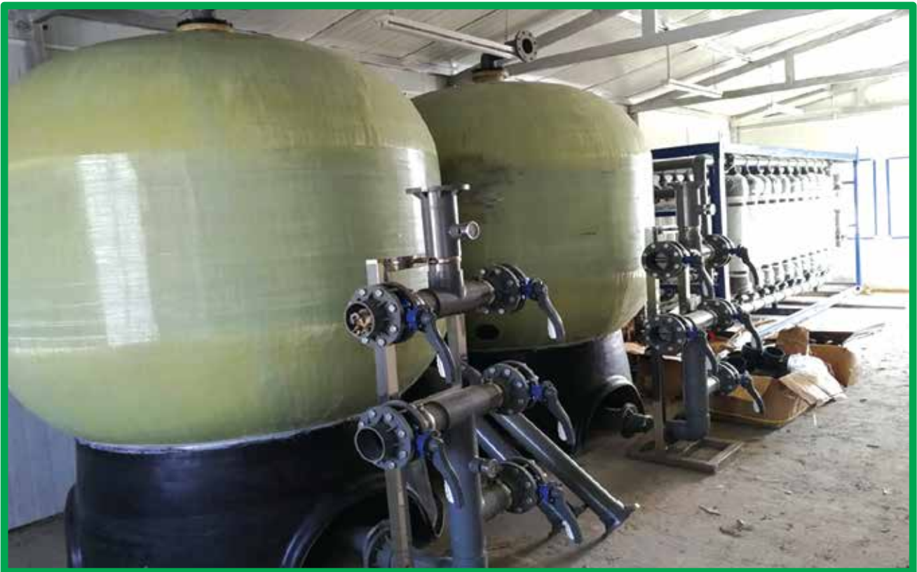
Water Treatment Facility at Project Site
