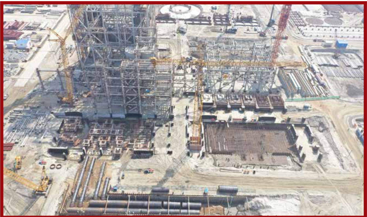
Turbine Hall Area
