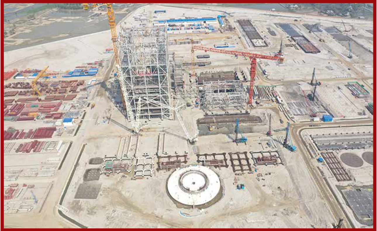
Boiler, Turbine, Generator Area
