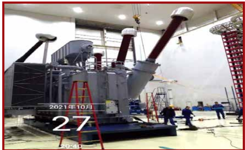
Generator Step Up Transformer
