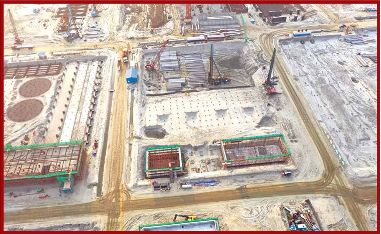
Water Treatment Area
