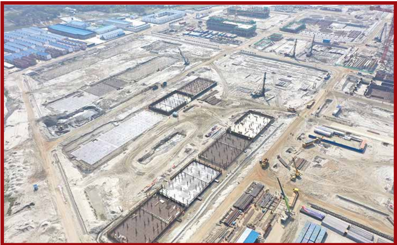
Induced Draft Cooling Tower Area
